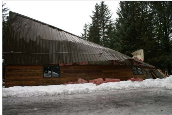
Seward Chapel Collapse
