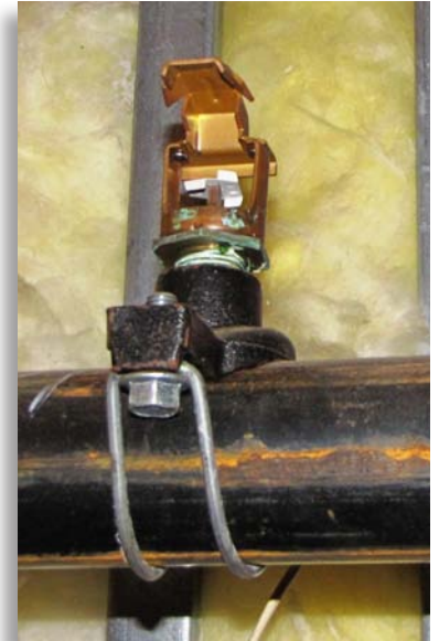
This attic sprinkler is one example of a “special sprinkler.”
