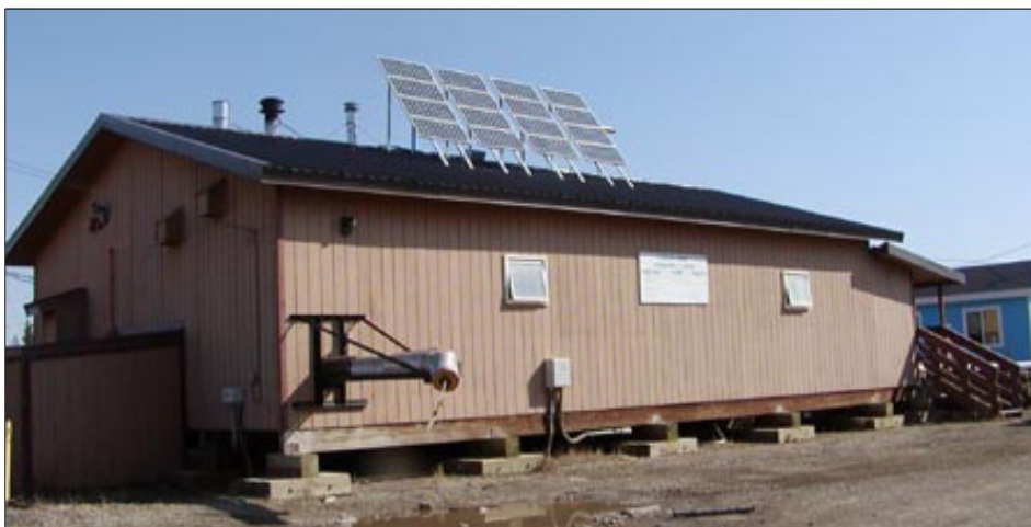
Solar panels have been used to augment power supply and act as emergency power for the school, clinic, and washeteria, shown here. The solar panels are more efficient than expected and the community hopes to expand the system in the near future.
