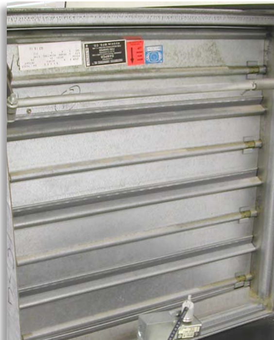
This smoke damper is closed to demonstrate its operational characteristics.
