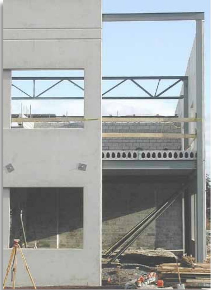
Concrete and steel are two important elements of this noncombustible building type, and may be required to have some fire resistance.
