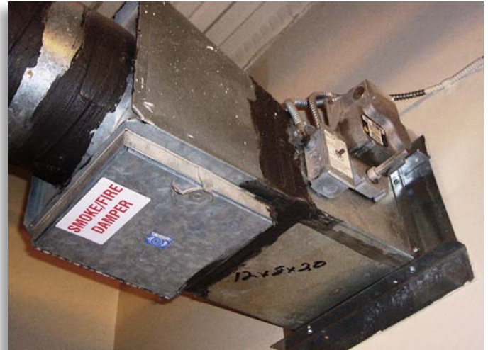
There is a combination smoke/fire damper behind this access panel. The actuator is nearest the wall at the upper right-hand corner of the picture.
