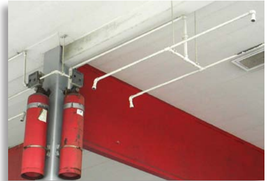
This dry chemical system beneath a service station canopy should be inspected by the owner monthly.
