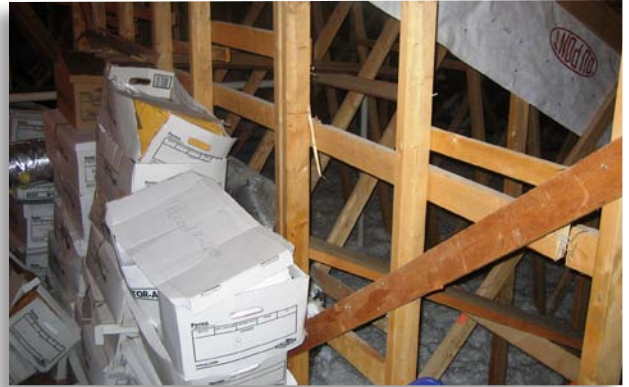
Attic storage like these boxes is prohibited by the fire codes except in specific cases.
