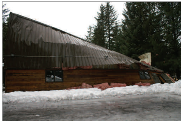
Seward Chapel Collapse
