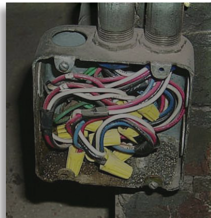
In addition to missing its required cover, this metal junction box appears to have too many conductors for its volume.
