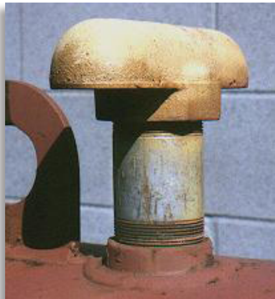
The vent outlet for this aboveground storage tank should be located at least 12 feet (366 cm) above the adjacent ground level.
