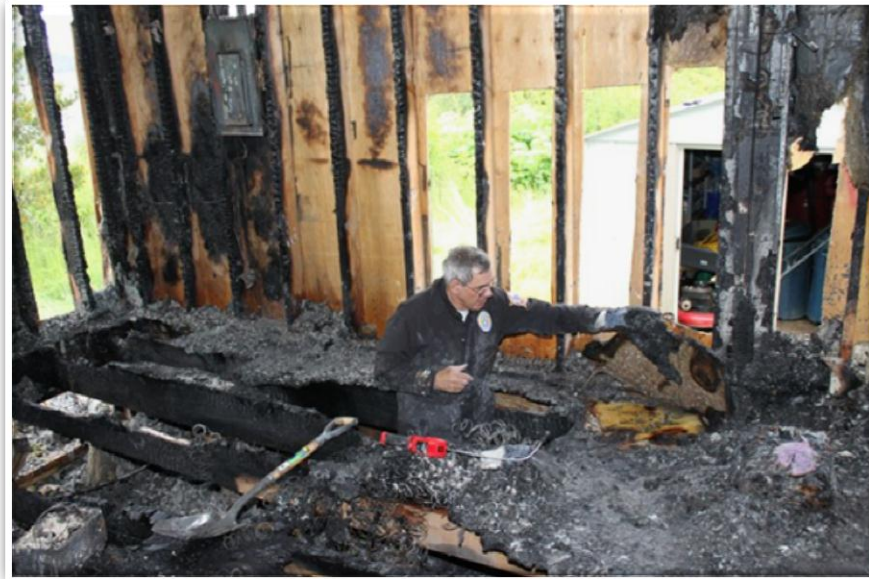
DFM, Bob Plumb (above) is working through fire debris to locate the fire of origin.
