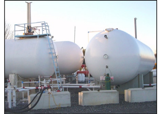
These bulk liquefied petroleum gas containers must meet minimum shell-to-shell spacing requirements.
