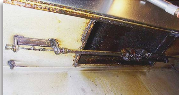
These fusible links likely are due for replacement since they are heavily coated in grease. Photo courtesy Jim Tidwell, Fire Equipment Manufacturer's Association.
