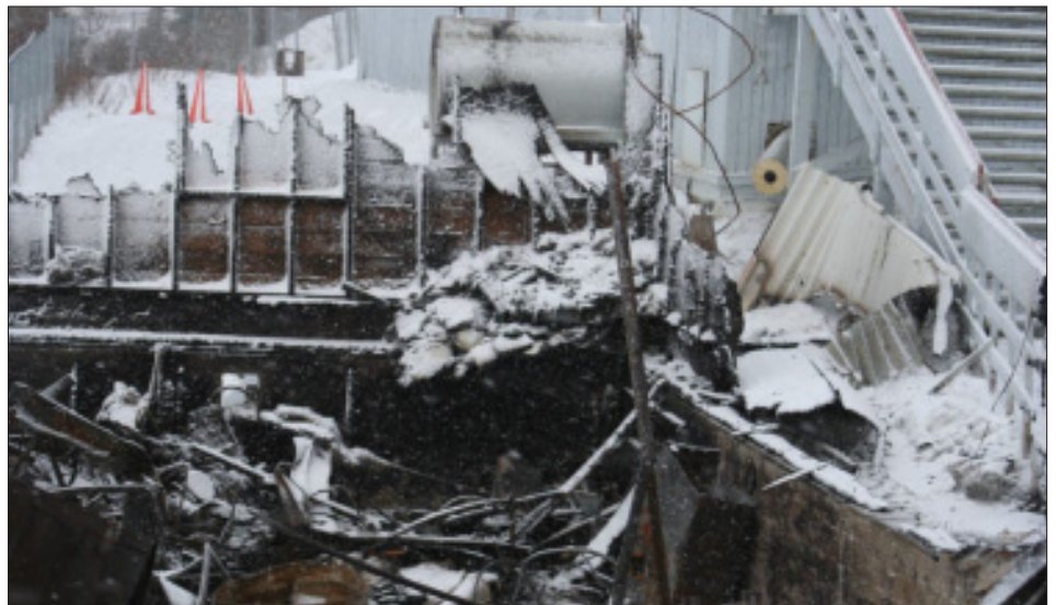
Following the fire at White Mountain School, the fuel tank, near the top center, shows it as virtually undamaged.
