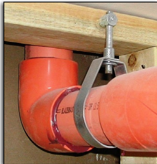
The hanger for this 3-inch (80 mm) pipe must be within recommended spacing limits.
