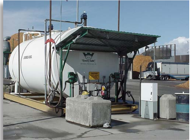
The dispensing area around this aboveground tank is a Class I location.
