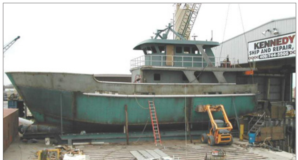
Enforcer II is under construction in Galveston, Texas. The anticipated launch date is in April.
