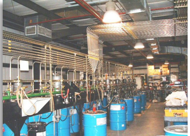
The electrical equipment in this flammable liquid dispensing room should be evaluated to ensure it is in compliance with the material group requirements of the National Fire Protection Association (NFPA) 70, National Electrical Code ® .
