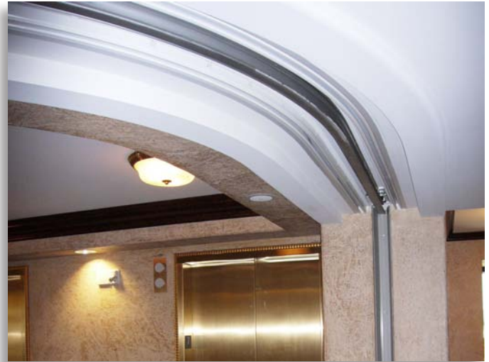
The curved track on the ceiling guides a motorized fire door used to create an elevator lobby.
