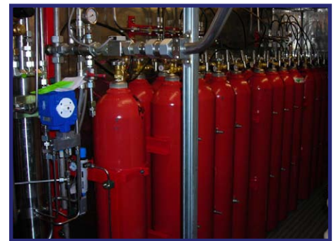
The Shungank School incorporates a non-electric gas driving pump for its fire protection.
