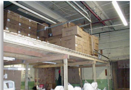
This "add on" mezzanine increases storage capacity, but requires automatic sprinkler protection beneath it. Photo courtesy of Martin M. King, West Allis, WI.
