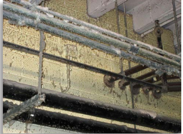
The accumulation of highly combustible lint in this commercial laundromat should cause the inspector to review the electrical classified location requirements.
