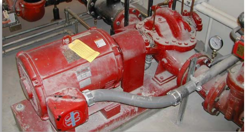
Electrically-driven fire pumps like this horizontal split case require a reliable power source to drive the pump.
