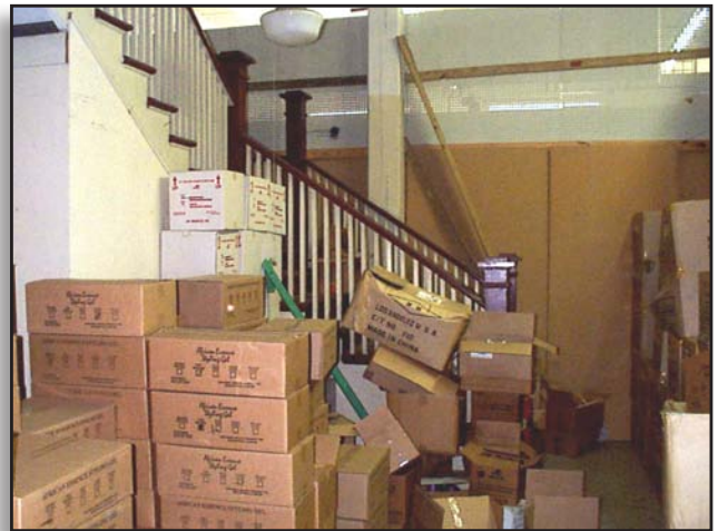
The accumulation of combustible material in this basement adds a substantial amount of fuel load to an area with limited ventilation and fire attack options.
